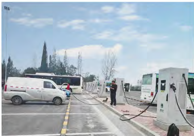
Changbai mountain public EV charging station in Jilin province, China
