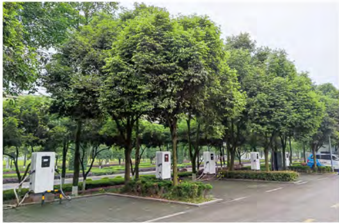
Public bus stop EV charging station in Chongqing, China
