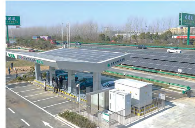
Highway service area PV+ESS+Charger station in Anhui province, China 🇨🇳
