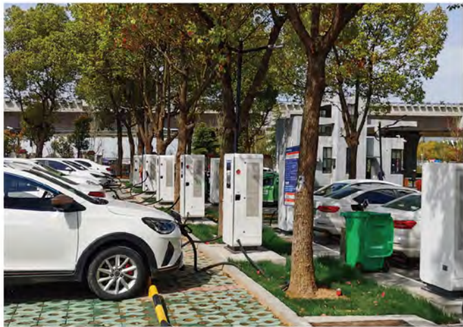
Qijian Technology EV charging station in Hefei, China
