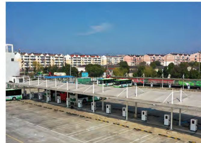
Chaohu public bus EV charging station in Hefei, China 🇨🇳
