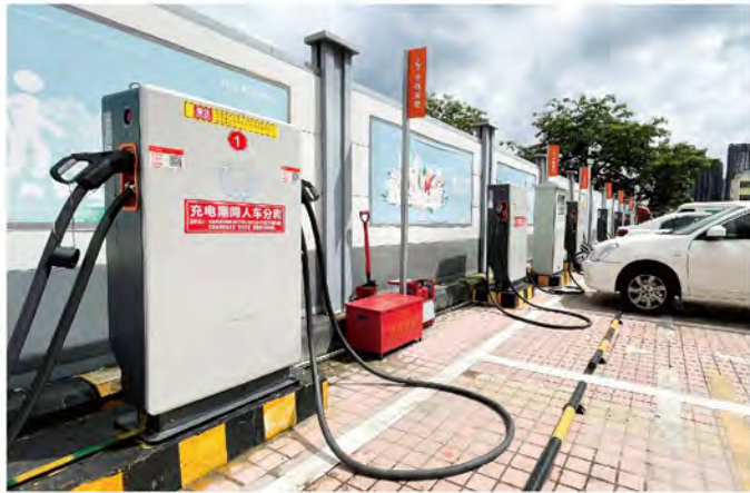
Huigangcheng EV charging station in Shenzhen, China
